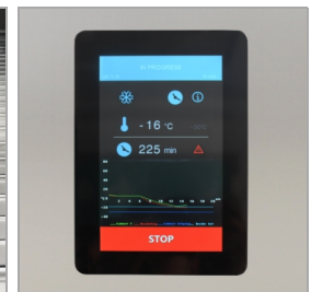
Touch screen controller
